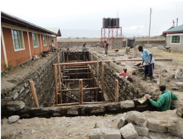
The underground tank.
